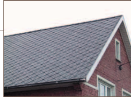
Dakleien in asbestcement
